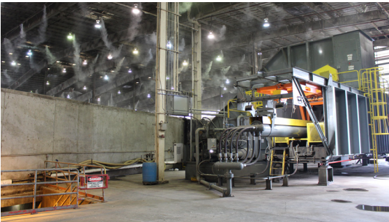
Machine for compacting waste materials into shipping container, DSNY Staten Island Transfer Station, Staten
